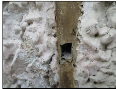
Photo N° 3189 ECH-N°12 -BAT 32-210 pignons Murs Joint de dilatation
