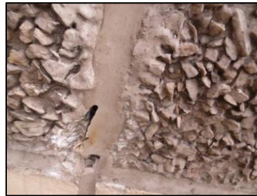
Photo N° 3193 ECH-N°15 -BAT 32-210 pignons Murs Joint de dilatation
